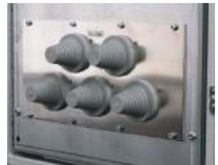
Cable routing through the divider panel of a Rittal TS8 baying enclosure system via module plates.
