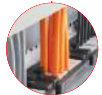
Straight cable routing into the cable duct
